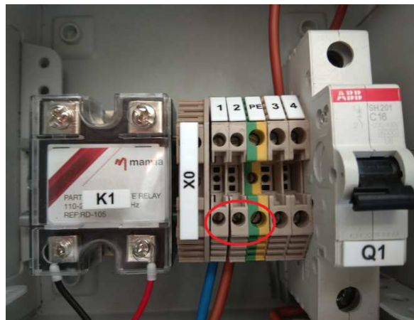
Power supply terminals block
